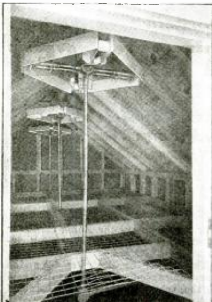
Here is shown the entirely new and unique 3-unit antenna installation for the runway localizer transmitters, of the new instrument-landing system, which radiates a horizontally-polarized "left-right" beam.
